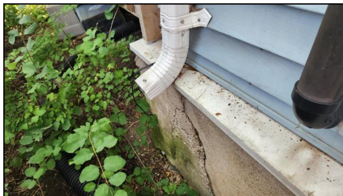
2. Should discharge 6 feet from building
