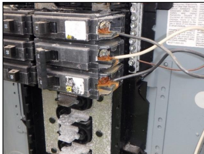
7. Rust or water in panel
