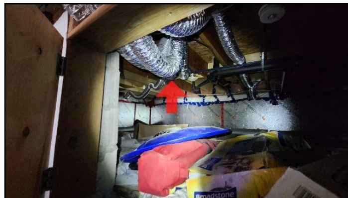
12. Excessively long runs, excessive elbows
