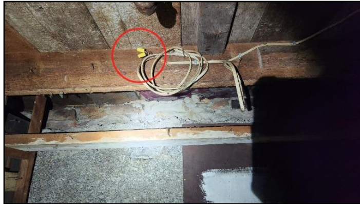
8. Missing junction box
