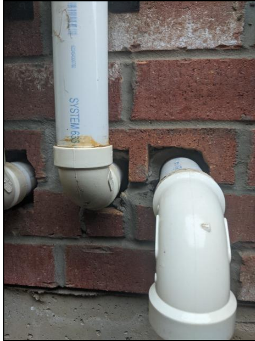
3. Caulking missing or ineffective
